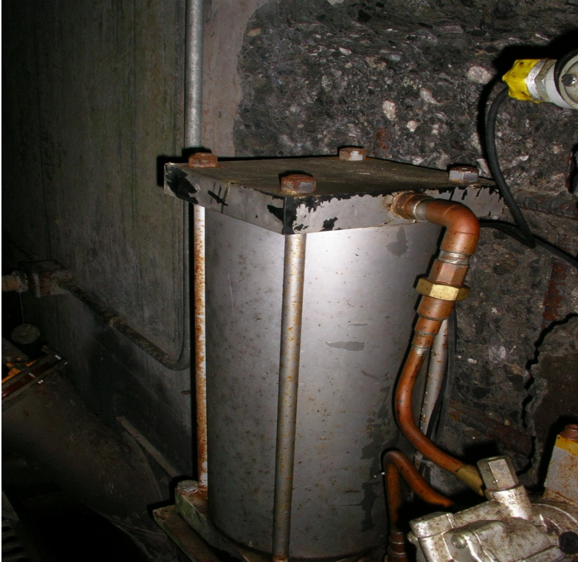
Photo 3-1. Grey Actuators with Concrete Chipped Away (Offset = 0.6 inches)
