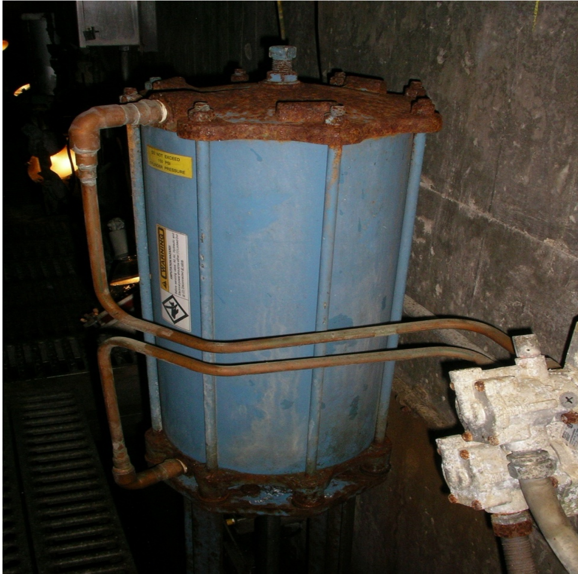
Photo 3-3. Blue Actuators with No Concrete Chipped Away (Offset = 7.2 inches)
