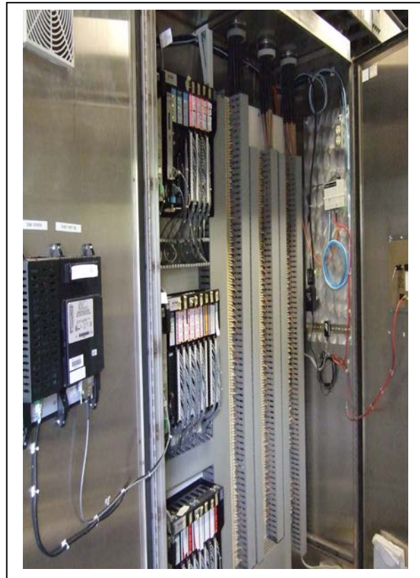
Figure 5-5. PLC Cabinet, Elect. Rm +90 Deck
