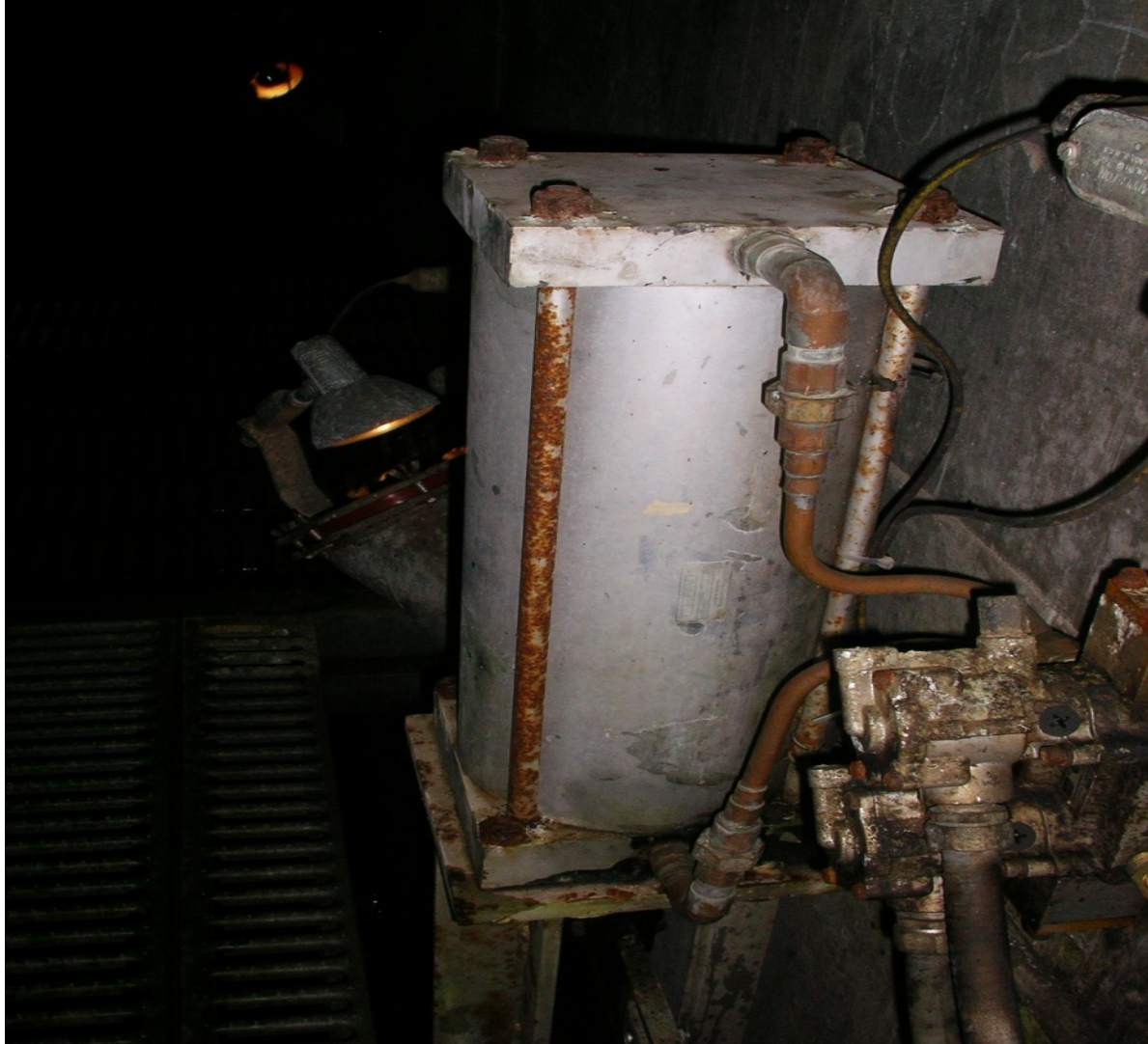
Photo 3-2. Grey Actuators with No Concrete Chipped Away (Offset = 4.2 inches)
